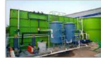
Sewage Treatment Plant Automation
