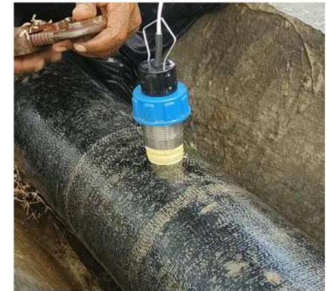
Paddle Wheel Flow meter Installation at KAHODA, GJ
